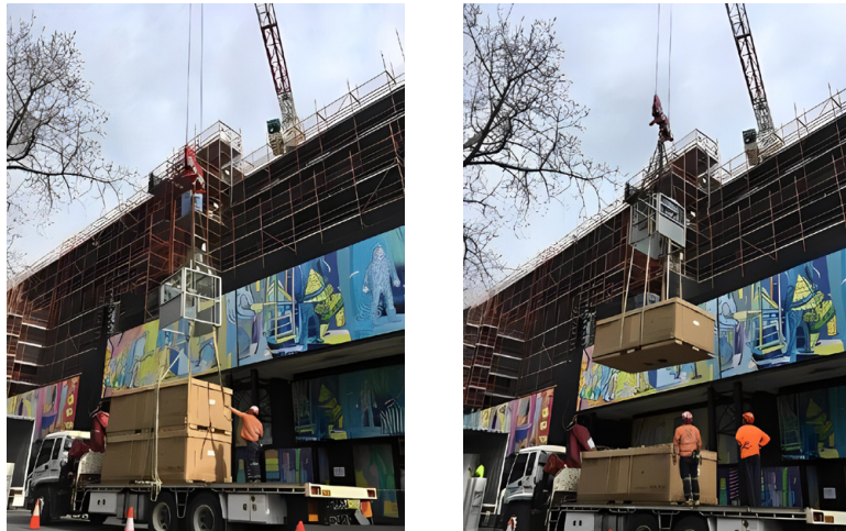
THE PICTURES ABOVE SHOW SATU BUMI PLANTERS, THAT EACH WEIGH JUST UNDER A TON, BEING SLING-LIFTED ONTO A HIGH-RISE BUILDING.
